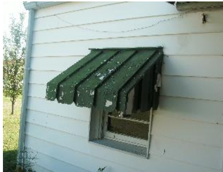
peeling paint on exterior awnings
