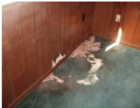
damaged and damp floor area in family room
