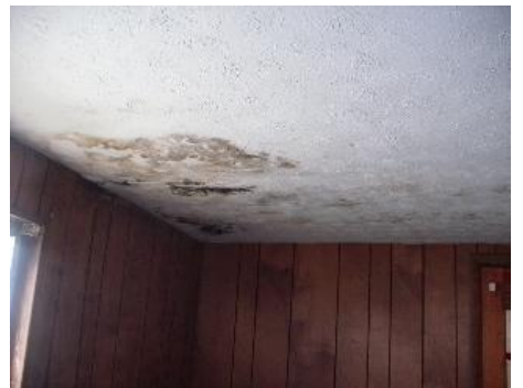
another ceiling damage area in family room
