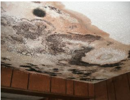
mold and ceiling damage in family room
