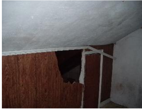
damaged area in 3rd bedroom
